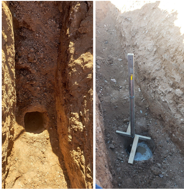
Figure 3-2: Typical test pit after excavation (right) and a test pit with ongoing infiltration test (left).
